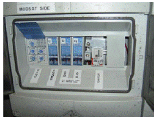
Weather station for controlling automatic curtain
